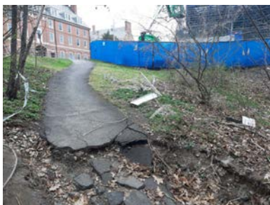
Steep, eroded path where it meets Paradise Road.
